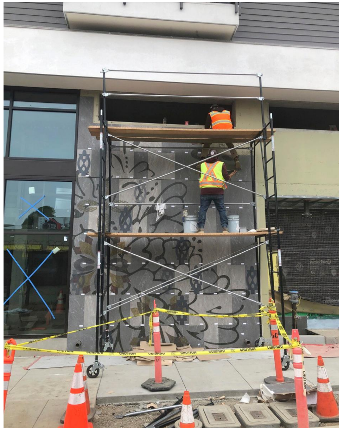
Ceramic tile by Julie Chang being installed at Webster Eleven on Harrison Street, Oakland, CA
